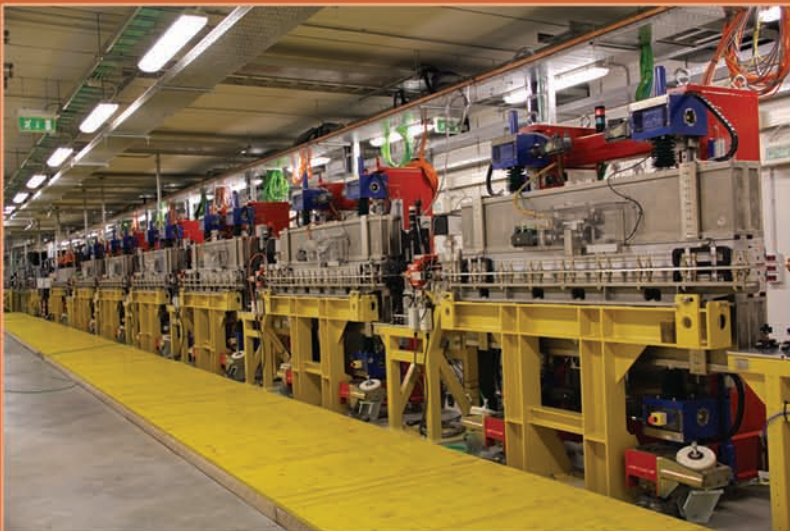
KYMA Elliptically Polarizing Magnetic undulator in the FERMI@Elettra tunnel
