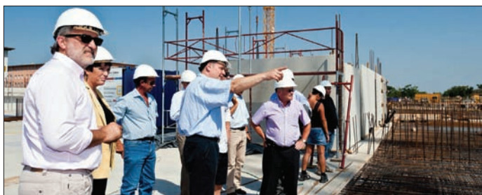
Michael Benedikt, centre, describes work on the MedAustron construction site to Steve Myers and members of CERN's accelerator management during a visit on 25 August 2011. (Image credit: Thomas Kästenbauer/Bildreport Austria.)
